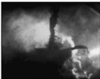
Initial venting and arcing.
